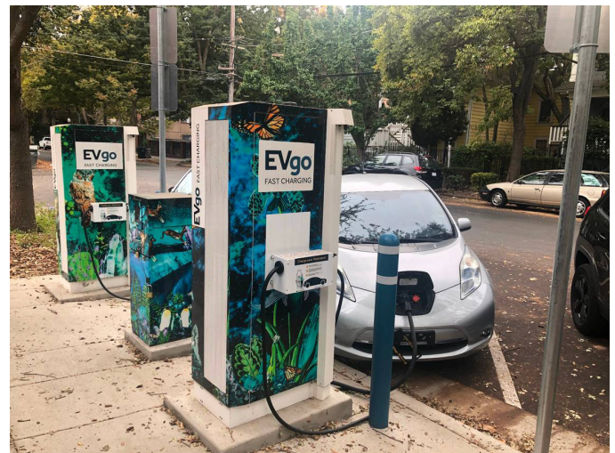
On-Street EV Charging in Sacramento Image Courtesy of the Sacramento Bee
